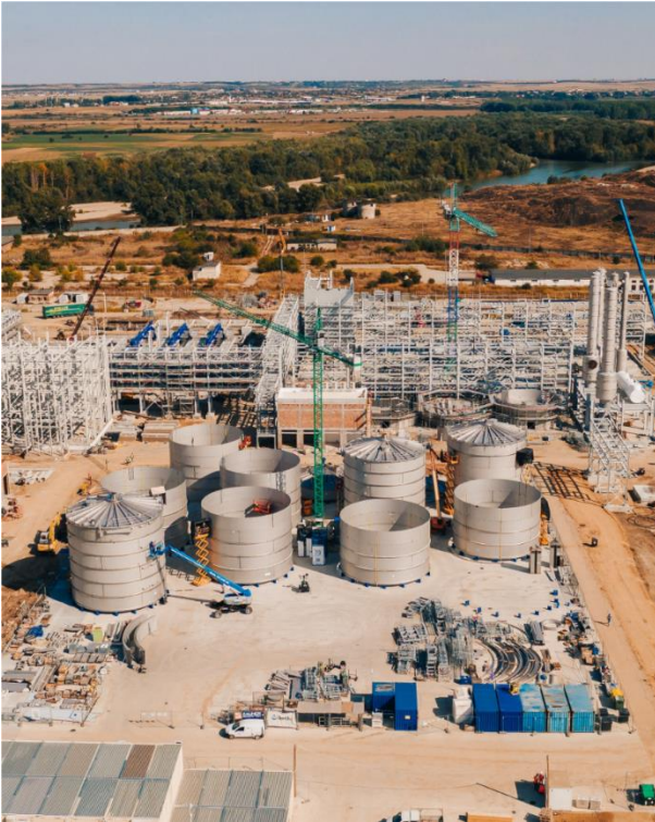
PICTURE CAPTION: CURRENT AERIAL VIEW OF THE CLARIANT SUNLIQUID® CONSTRUCTION SITE IN PODARI, ROMANIA (PHOTO CREDITS: CLARIANT)
